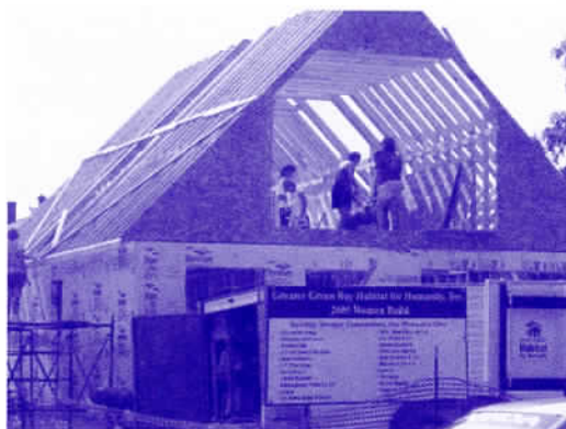
Laying the upstairs floor boards at the Greater Green Bay Habitat for Humanity 2005 Women Build.
